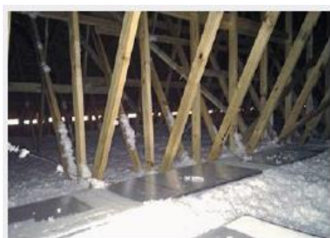
After attic insulation was installed (shown), additional R-30 insulation was mounded above the ducts.
