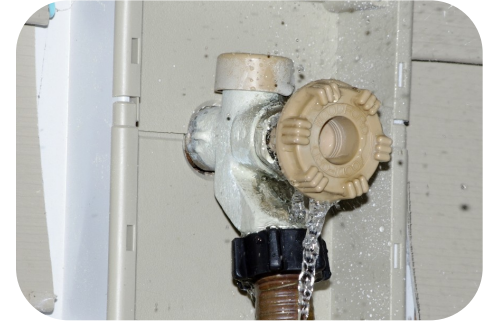
Leaks/Other Water Use
